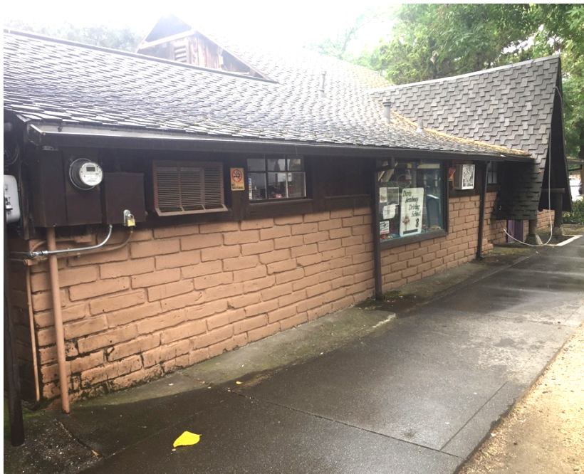
Figure 1. North elevation of 340 G Street viewed from sidewalk along 4th Street, looking southwest.
